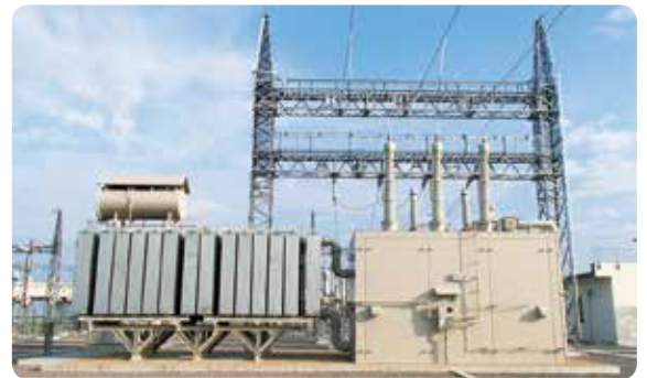
Shin-Hakodate Transformer Substation
