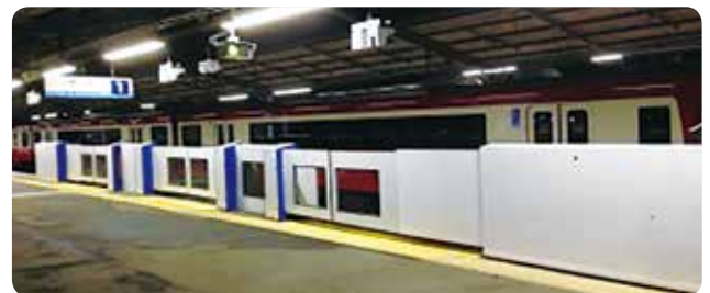
Platform edge doors (Mitsubishi Heavy Industries Transportation Equipment Engineering & Service Company)
