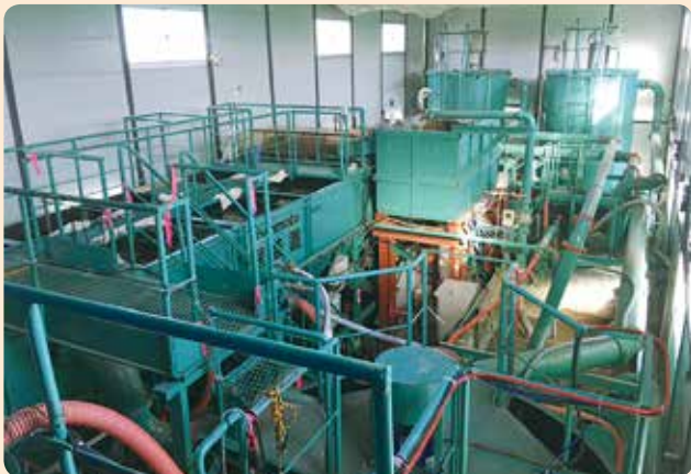
Turbid water treatment equipment
