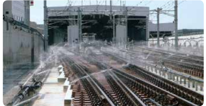
Snow removal sprinklers (Hokuriku Shinkansen)
