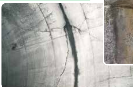
Cracks inside a tunnel
